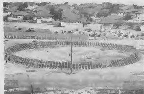
THE FRAME is up, the foundation is placed. All this took place after careful surveying and leveling of the site.
